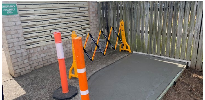
Queen Street residents can now collect their copies of the Village Voice from the mail centre more smoothly thanks to the new concrete extension.
