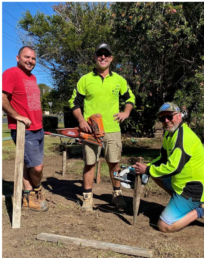
On the home straight: the NJS Construction team Rio Grieves, Nat Sewell, and Jason Skinner are nearing completion of the Stage 2 footpaths.
